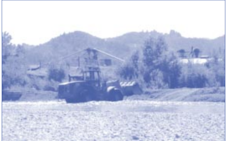
Shamrock was allowed by NOAA Fisheries and DF&G to drive this 30 ton loader across the river in two places twice a day, for a total of over 40 crossings. Their permit allows only 10 wet stream crossings per year!
